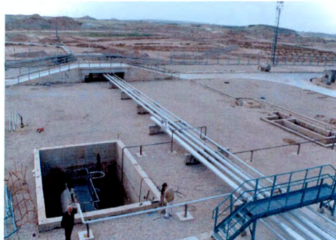
محوطه H/C Closed Drain Pit , Oily Water Separator
